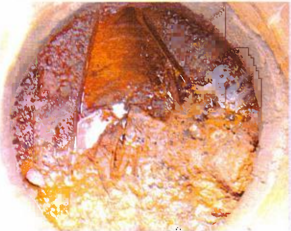
Main Post – MH 9E (Riverside Avenue) Estimated 2 gpm (3,000 gpd) from caps of both pipes.
