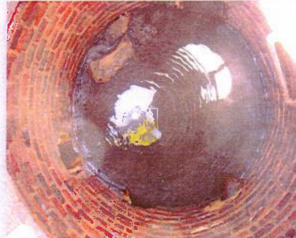
Charles Wood – MH 9 (Guam Lane) View of 4-inches stagnant flow. Manhole appears to have no channel.
