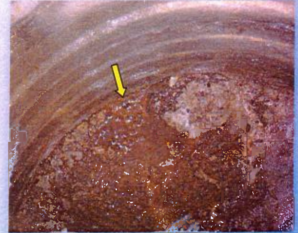
Charles Wood – MH 46 (Corregidor Road) Arrow points to estimated 3 gpm (4,300 gpd) from wall and bench junction.
