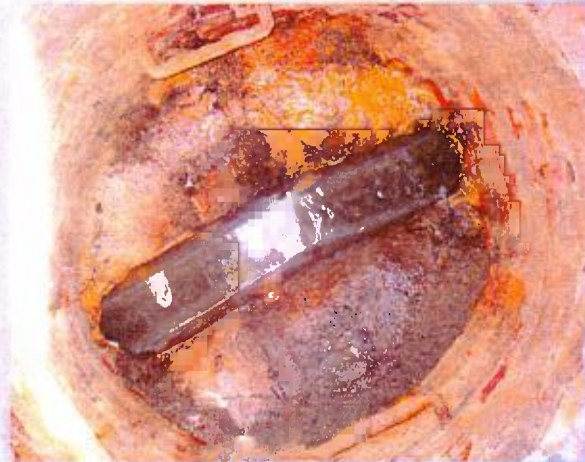
Main Post – MH 21 (Barkers Circle) Estimated 2 gpm (3,000 gpd) from sleeve of effluent pipe, benching, and wall and bench junction.
