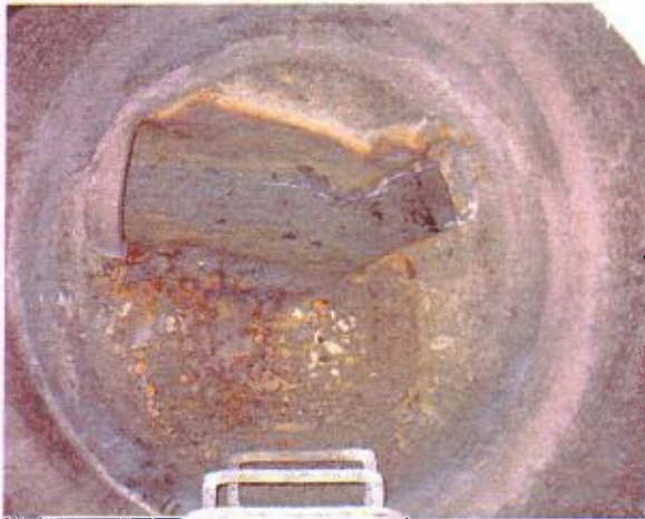
Charles Wood – MH 1A (Guam Lane ROW) Minor hydrogen sulfide (H 2 S) corrosion observed on manhole walls and riser.
