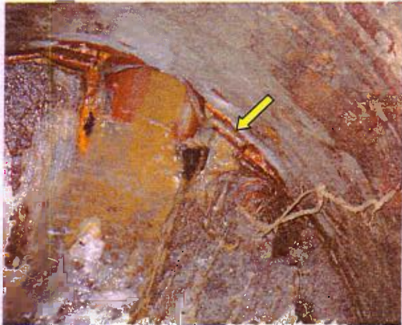
Charles Wood – MH 44B (Hemphill Road) Arrow points to estimated 2 gpm (3,000 gpd) wall leak to right of effluent pipe. Minor root intrusion from wall / bench junction.
