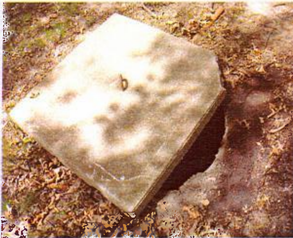
Main Post – MH 15A (Barkers Circle) View of concrete slab placed over manhole; no frame or rim on manhole. HMM unable to remove slab.
