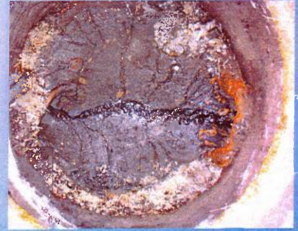
Main Post – MH 144 (Sherrill Avenue) View of significant hydrogen sulfide (H 2 S) corrosion throughout manhole.
