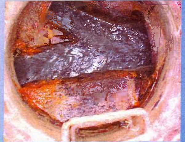
Main Post – MH 59 (Allen Court) Estimated 1 gpm (1,500 gpd) from the sleeves of both influent pipes.
