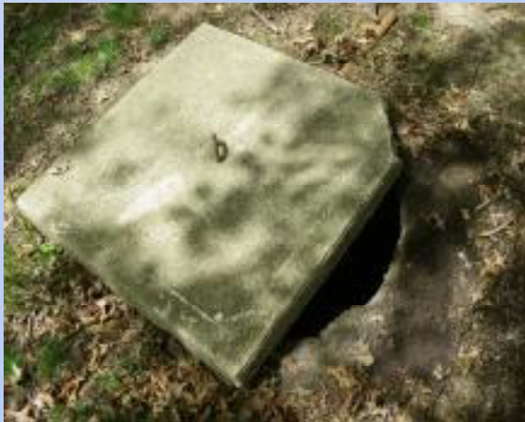
Main Post – MH 15A (Barkers Circle) View of concrete slab placed over manhole; no frame or rim on manhole. HMM unable to remove slab.
