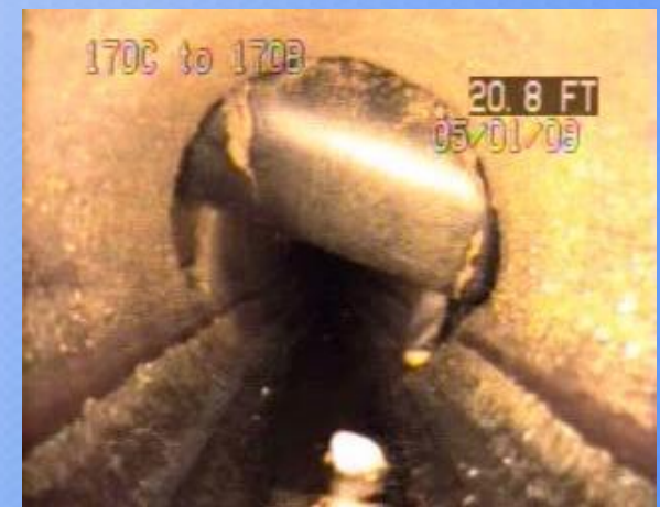
MH 170C to 170B – Avenue of Memories View of unknown utility pipe crossing through sanitary sewer 22 LF from MH 170C.
