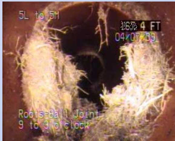
Charles Wood: MH 5M to 5L – Megill Drive Joint with 30% root mass (indication of leak) 167.4 LF from MH 5L.
