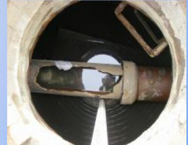
Charles Wood – MH 23 (Heliport ROW) View of doghouse manhole with unenclosed pipe. Survey rod used to measure 12-inches of stagnant flow.
