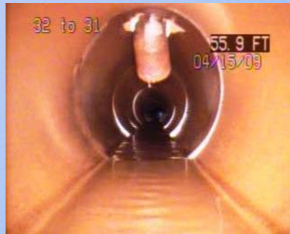
MH 32 to 31 – BLDG 2700 PBSC protruding 6-inches into mainline 60.4 LF from MH 32.
