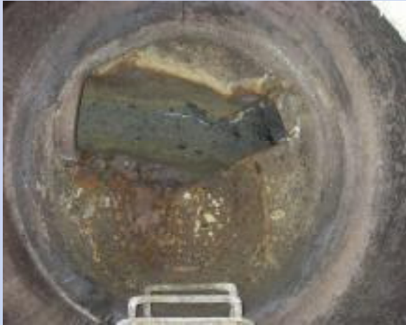
Charles Wood – MH 1A (Guam Lane ROW) Minor hydrogen sulfide (H 2 S) corrosion observed on manhole walls and riser.
