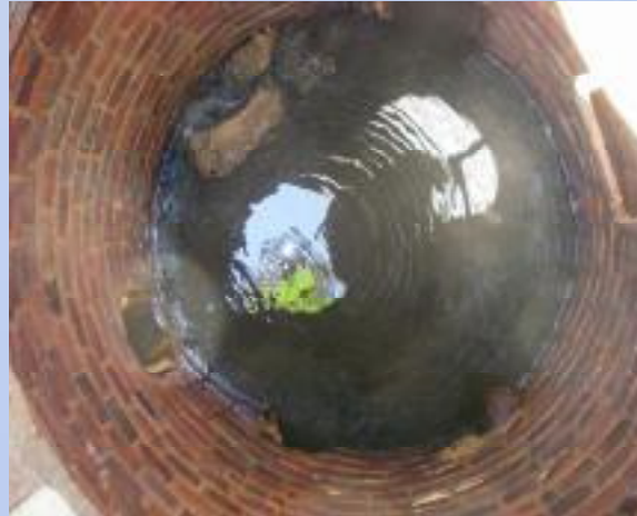
Charles Wood – MH 9 (Guam Lane) View of 4-inches stagnant flow. Manhole appears to have no channel.
