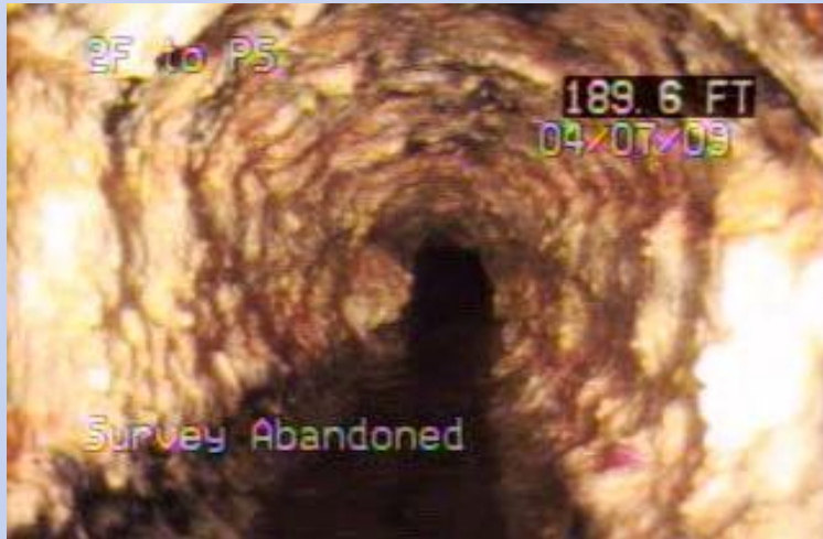
Charles Wood: MH 2F to PS - Club House Area Grease accumulation (25%) 189.6 LF from MH 2F.
