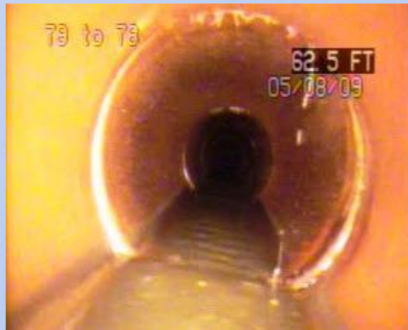
Main Post: MH 79 to 78 – Easement Estimated 150 gpd from joint 64 LF from MH 79.
