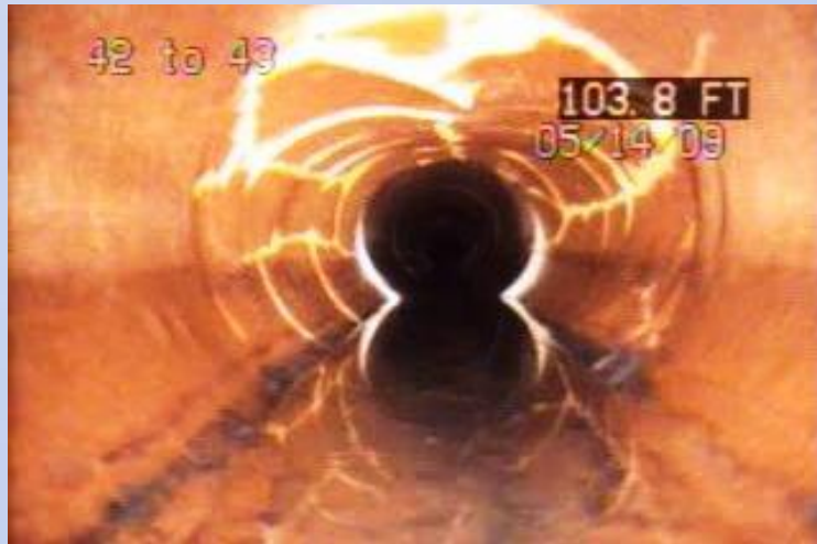
MH 42 to MH 43 - Apex Avenue Grade 4 fractured pipe section with 15% loss of ovality.
