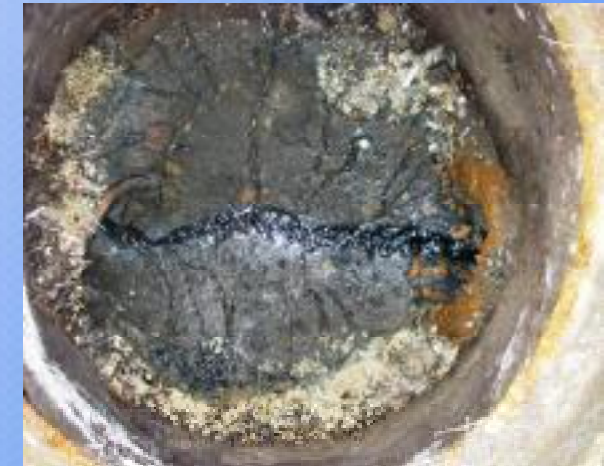
Main Post – MH 144 (Sherrill Avenue) View of significant hydrogen sulfide (H 2 S) corrosion throughout manhole.
