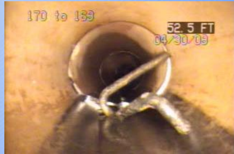
Main Post: MH 170 to MH 169 – Derum Avenue View of manhole run stuck in pipe.
