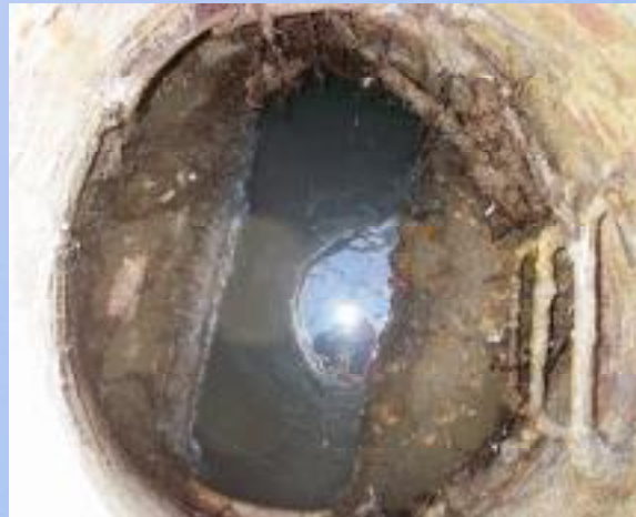
Main Post – MH 68 (Parkers Creek ROW) View of large root throughout manhole protruding from lower wall.
