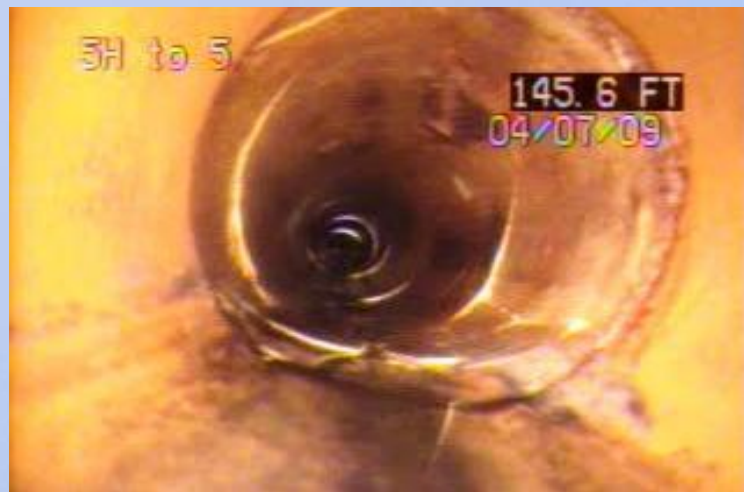
MH 5H to MH 5 - Megill Circle Grade 4 fractured pipe section 145.6 LF from MH 5H.
