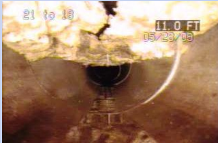
Main Post: MH 21 to MH 18 – 1 st Avenue Grease accumulation (30%) along pipe crown.
