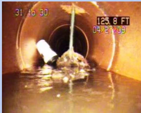
MH 31 to 30 – BLDG 2700 Easement View of metal bar protruding through mainline 128 LF from MH 30 trapping debris.
