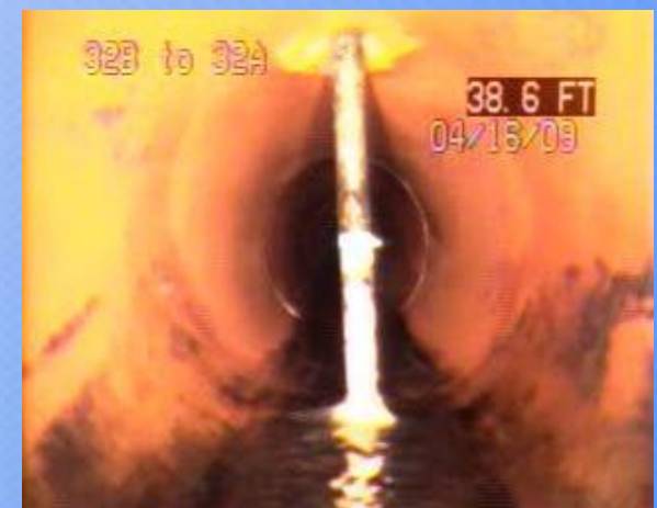
MH 32B to 32A – BLDG 2700 View of metal bar protruding through mainline 39.9 LF from MH 32B.
