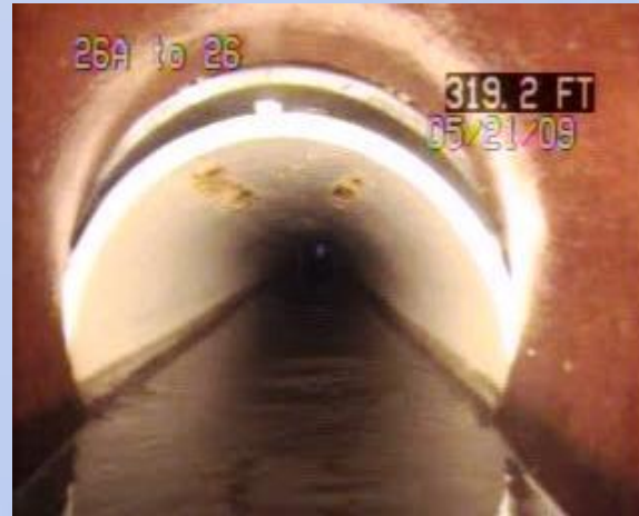
MH 26 A to 26 – Alley View of camera entering 50% pipe sag due to offset joint 320.3 LF from MH 26A.
