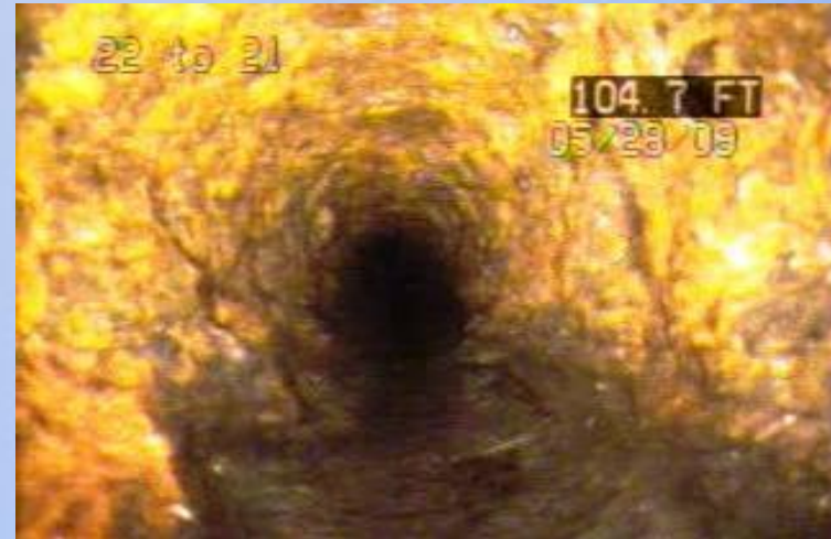
Main Post: MH 22 to MH 21 – 1 st Avenue Heavy tuberculation 103.6 to 129 LF from MH 22.
