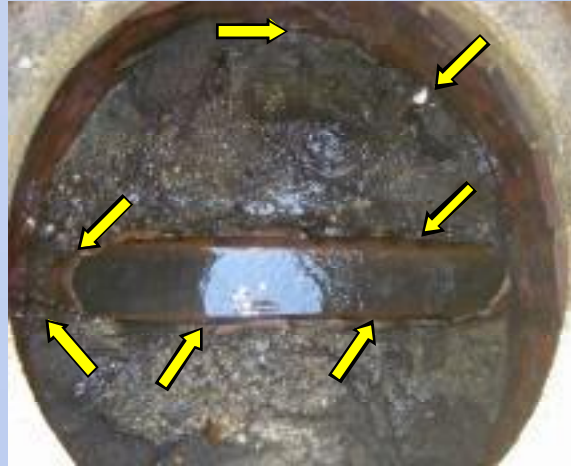
Charles Wood – MH 14 (Satellite Road ROW) Arrows point to estimated 7 gpm (10,100 gpd) from both pipe sleeves, wall / bench junction and benching.
