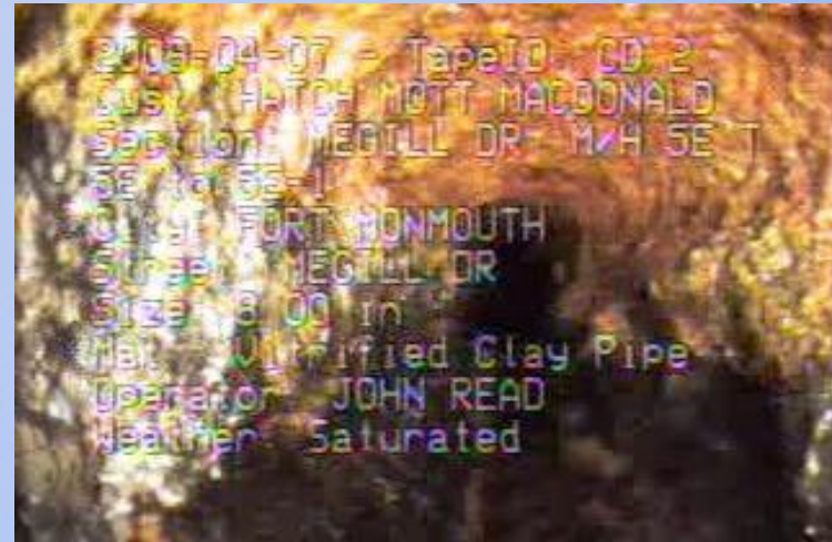
Charles Wood: MH 5E-1 to 5E – Megill Circle Heavy tuberculation throughout sewer.
