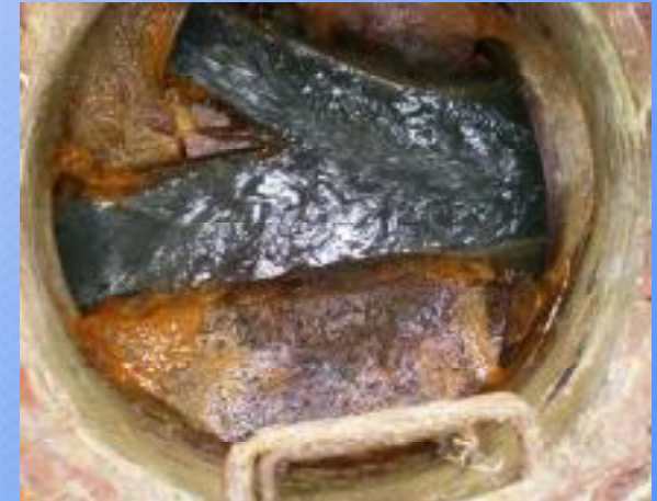
Main Post – MH 59 (Allen Court) Estimated 1 gpm (1,500 gpd) from the sleeves of both influent pipes.
