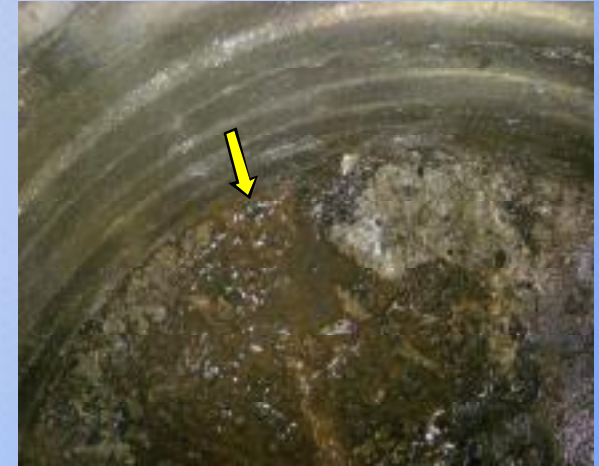
Charles Wood – MH 46 (Corregidor Road) Arrow points to estimated 3 gpm (4,300 gpd) from wall and bench junction.
