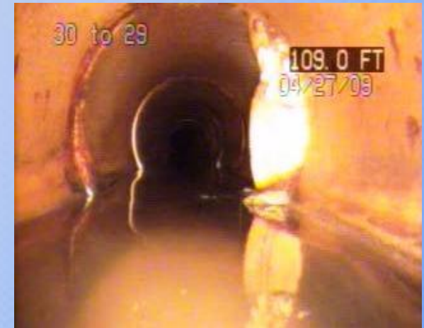
MH 30 to 29 – BLDG 2700 Easement PBSC protruding 2-inches into mainline 113 LF from MH 30.
