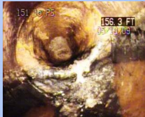
MH 151 to PS – Avenue of Memories View of pipe offset 6-inches at pipe material change junction 159.2 LF from MH 151.
