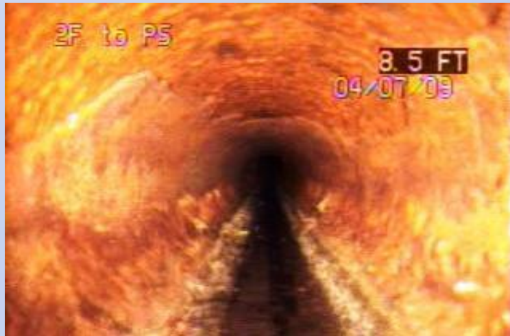
MH 2F to PS - Club House Area Grade 3 to 4 Hydrogen sulfide corrosion throughout sewer.
