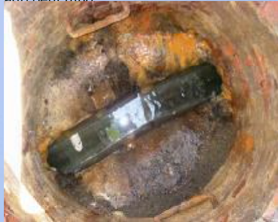
Main Post – MH 21 (Barkers Circle) Estimated 2 gpm (3,000 gpd) from sleeve of effluent pipe, benching, and wall and bench junction.
