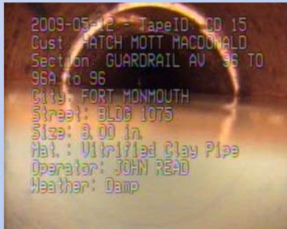
MH 96A to 96 – BLDG 1075 View of 50% sag from MH 96A to 15.1 LF downstream.
