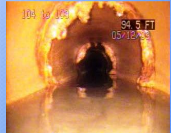
Main Post: MH 104 to 103 – BLDG 702 View of intermittent joints with mineral deposits.
