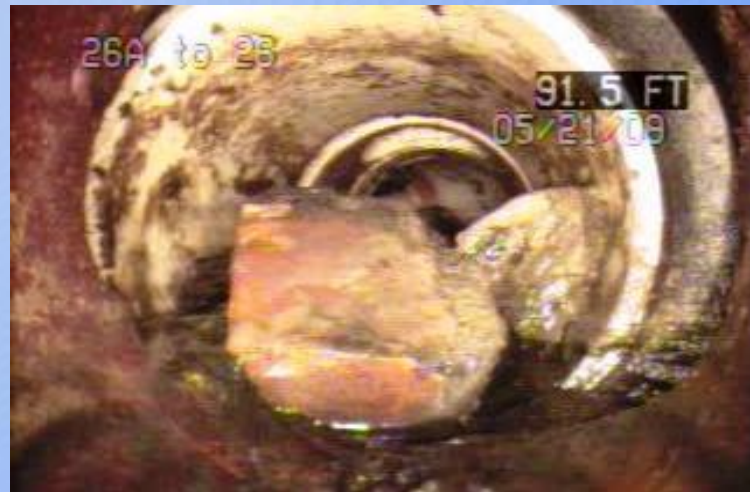
Main Post: MH 26A to MH 26 - Alley Rocks stuck in PBSC 91.5 LF from MH 26A.
