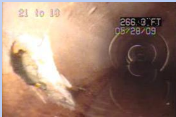
MH 21 to MH 18 - 1st Avenue Grade 5 hole with outer soil and rocks visible.
