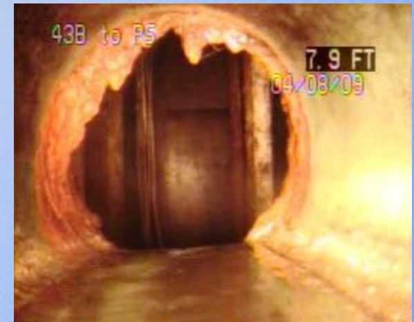
Charles Wood: MH PS – Hemphill Road Sleeve leak at influent pipe (150 gpd).
