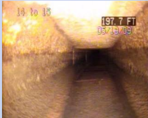
MH 14 to 15 – BLDG 208 Easement Pipe changes shape from circular to rectangular 197.3 to 212.3 LF from MH 15.
